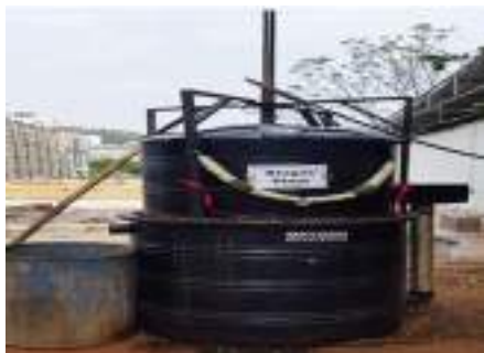
Figure 6.2.18 Bio Gas Plant
