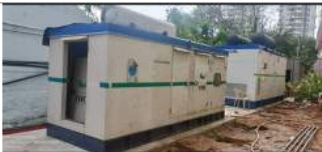
Figure 6.2.19 Power House Generators
