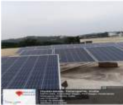
Figure 6.2.16 Solar Roof Top Power Plant
