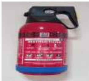
Fig. 6.2.15 Fire Extinguishers are installed in the Laboratory
